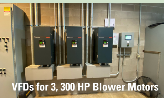
300 HP Blower Motor
