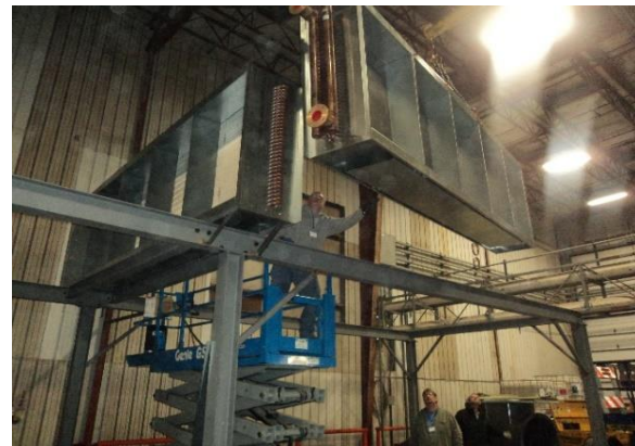
Scrubber Exhaust Heat for Makeup Air Preheating
