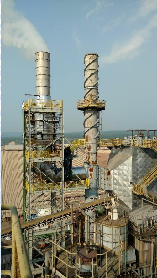
Wood-Fired Boiler Exhaust Heat Recovery
