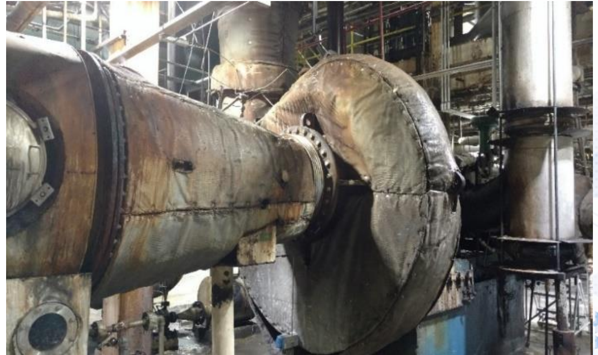
2,500 HP MVR Evaporator (Electric Semi-open)
