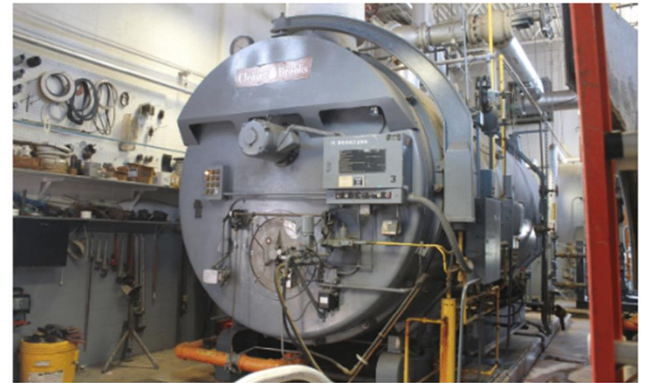
Image 2: 4 Pass 1960s firetube steam boiler
